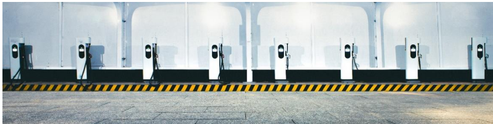
Figure 1: Electric Car Charging Stations
